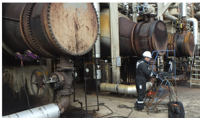
Heat exchanger, in-service corrosion mapping
